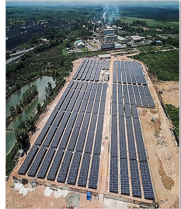
Installation completed of 3MW solar power PV plant with battery storage capacity of 2MW at Indominco
