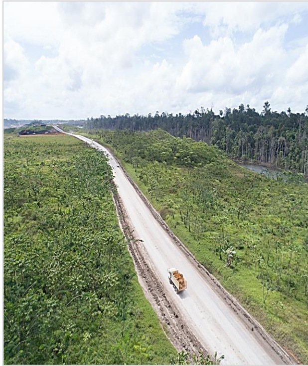
Completion of road infrastructure upgrade with bridges and road reaching 100 km connecting Trubaindo and Bharinto
